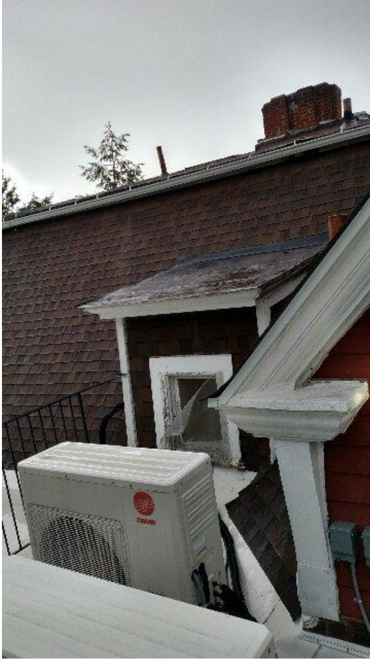
Exterior before – third floor fire escape access only.
